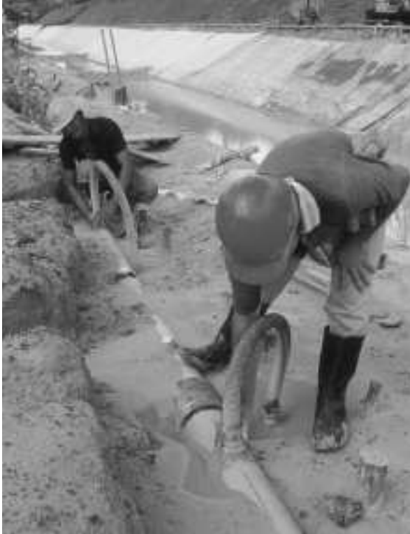
Set up pipes for the installation network Photo from World Bank Photo Library
